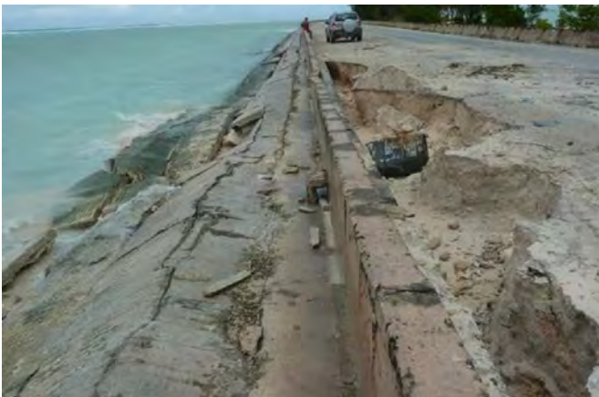
Damage to revetments and roads caused by king tides
