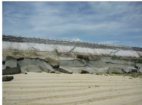
Damage to revetments (concrete mats)
