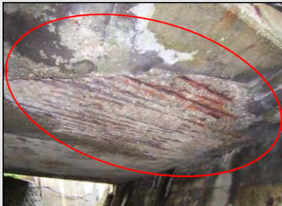
Concrete Bridge: Maintenance is very difficult
