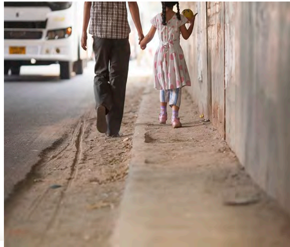
Footpath condition in Bangalore, India
