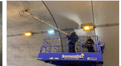
Radar to monitor deformation of tunnel lining
