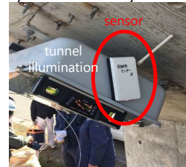
Monitoring sensor on tunnel facility
