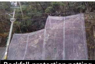
Rockfall protection netting
