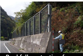
Rockfall protection fence
