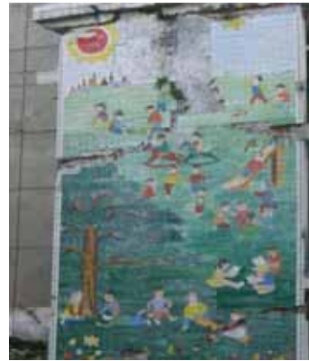
Fig.5 The mural of the kindergarten in the town of HanWang, photographed immediately after the catastrophe. Thanks to donations, it was reconstructed in spite of serious damage to the building.
