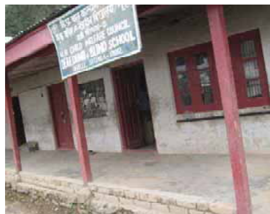
Fig. 2 Students' dormitory before the retrofit
