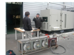
Gas Engine Generation
