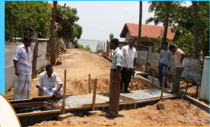
Process in operation
