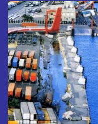
Container berth with a large crack
