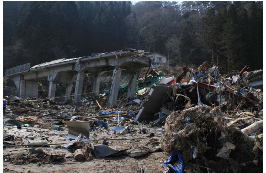
Wreckage of Bridge (North-Rias Line)
