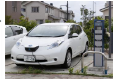
Two EVs are reserved. In case of an emergency, the V2H system supplies electricity to the assembly room, etc.
