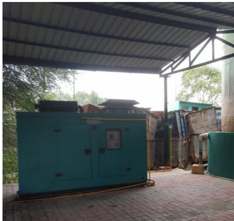
5. 100% biogas-fed engine for power generation
