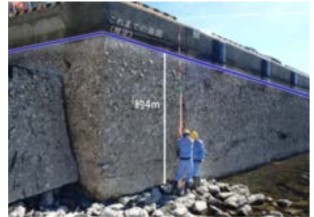
Lifted up by Earthquake
