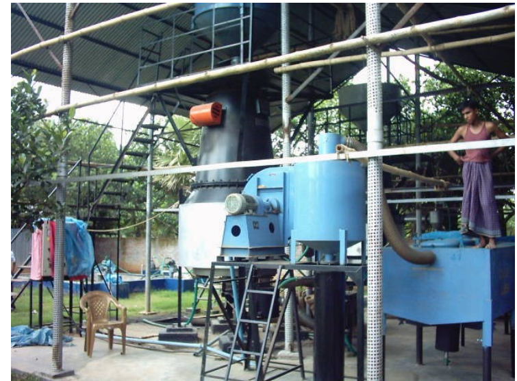
Bio-gas generation units; ladder shown used for feeding rice-husks
