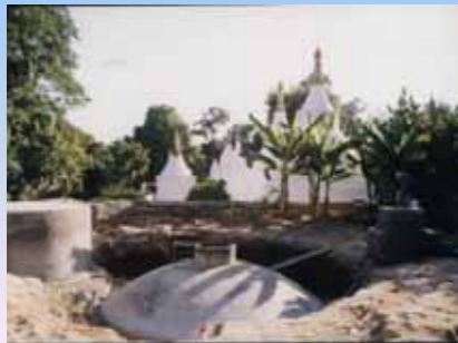
Fixed dome type biogas plant
