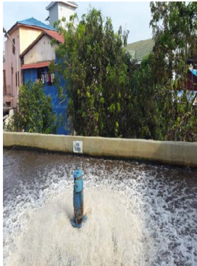
Margasari Wastewater Treatment Installation
