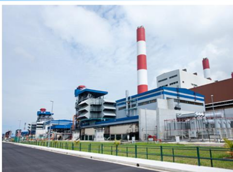
The picture shows the PowerSeraya's Combined Cycle Power CoGeneration Plant in Singapore. (Press picture: PowerSeraya)
