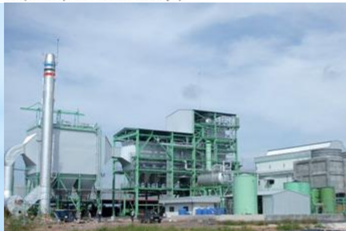
Biomass power generation facility using palm fruits bunch as fuel in Thailand (Source from MEIDENSHA CORPORATION)
