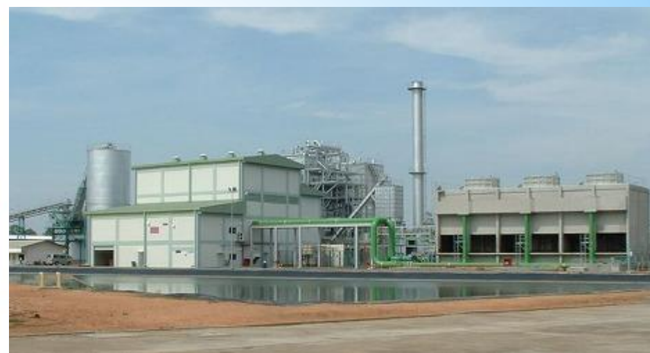
Biomass power generation facility using rice husks as fuel in Thailand (Source from MEIDENSHA CORPORATION)
