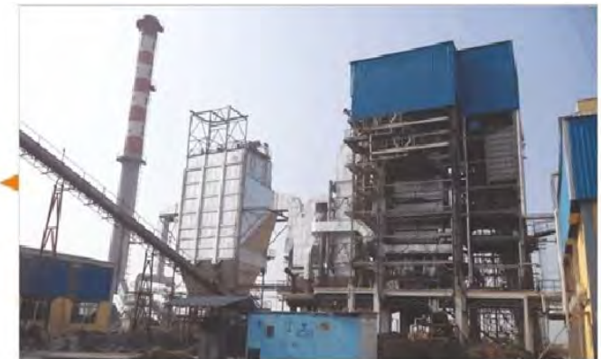
10 MW Grid Connected Biomass Power Plant at Thimmapur Village, Dist. Haveri
