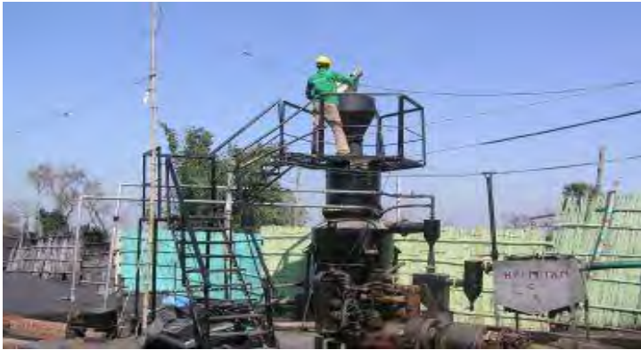
Filling gasifier plant with rice husk, Tamkuha.
