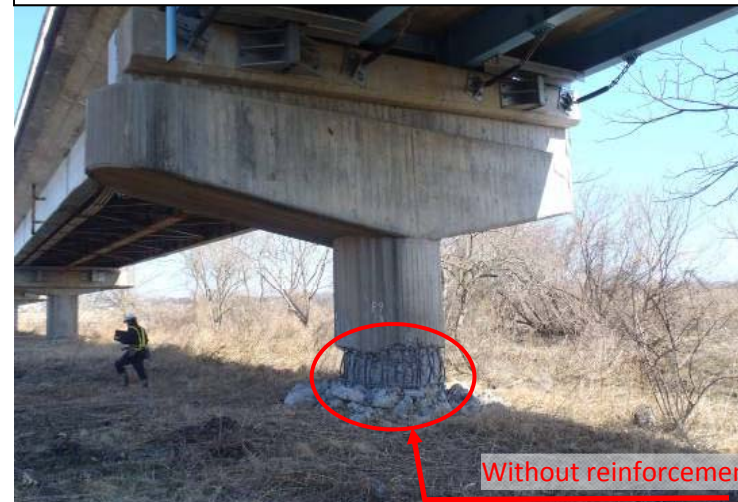
Prefectural road (Observed intensity: 5-)
