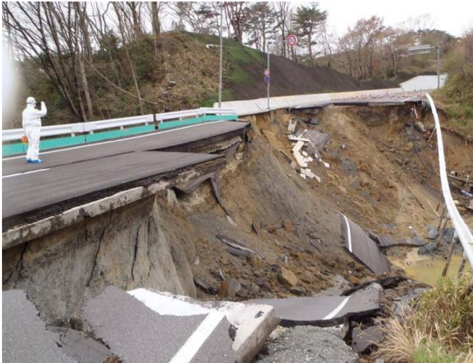
Soon after the earthquake, on March 11, 2011
