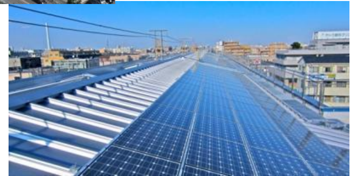
Photovoltaic generation system
