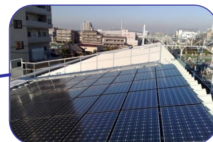
Photovoltaic generation system
