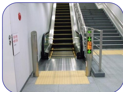
Automatically operated escalators
