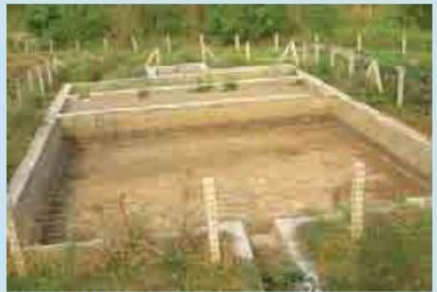
Leachate collection tank
