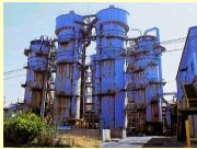
Flue gas desulfurization system
