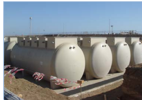
Employee dormitory (Saudi arabia: 530\text{m}^3/\text{d} )
