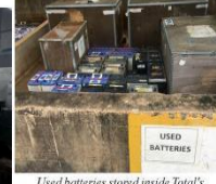
Used batteries stored inside Total's pipeline centre
