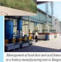
Management of lead dust and acid fumes in a battery manufacturing unit in Yangon
