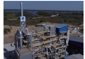
Waste-to-energy facility constructed by a Japanese firm in Yangon, Myanmar
