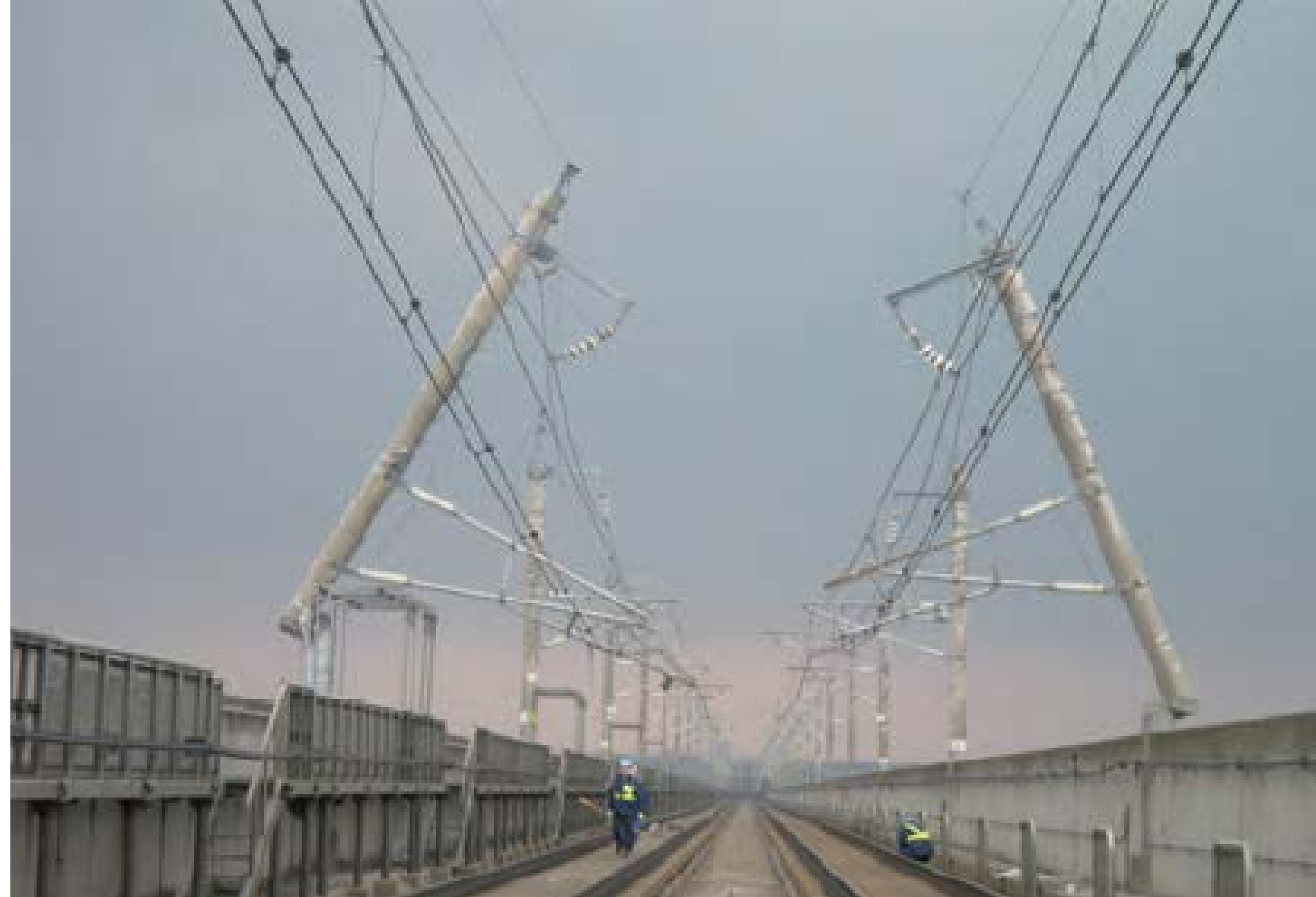
After Great East Japan Disaster in 2011, Shinkansen Stopped for 49 days mainly because of electric poll destruction (photo by JR east)
