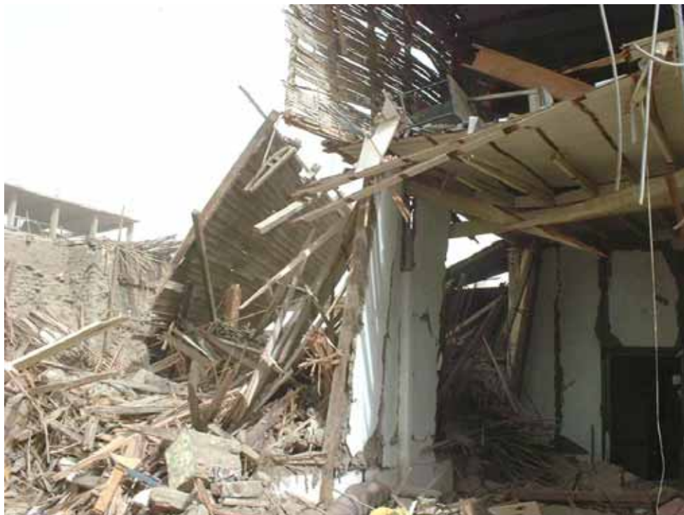
Photo 2: Destruction of quincha in Pisco, Ica Province
