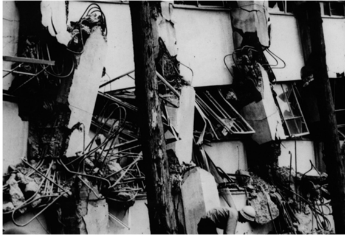
Photo 4: The Hakodate Technical University building collapsed after the 1968 Tokachi-oki Earthquake
