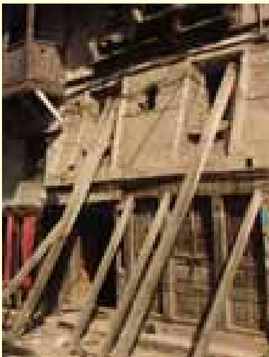
Photo 3: Old houses with cracks and electric wires
