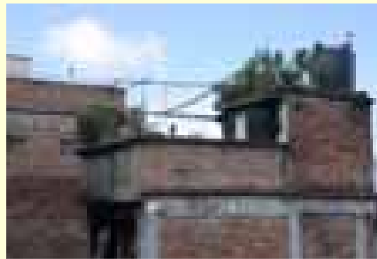
Photo 2: Installation of water tanks on the top floor without protection
