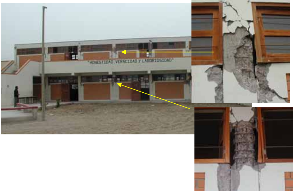
Photo 6: Damaged schools built with 1977 Standard (Photos: E. Fierro)
