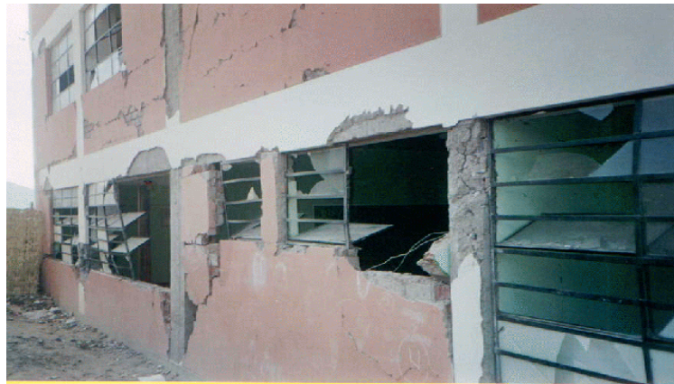
Photo: 5: Damaged classrooms
