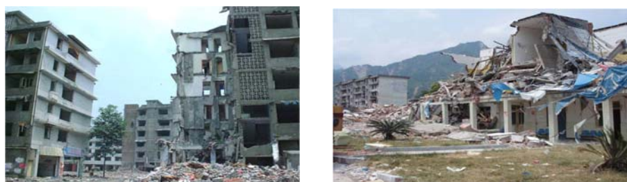
Figure 11. Damages in Middle Storey Apartment Houses- 5-6 Storeys Buildings (Left), Hospital in Hanwang (Right), Sichuan Province, China
