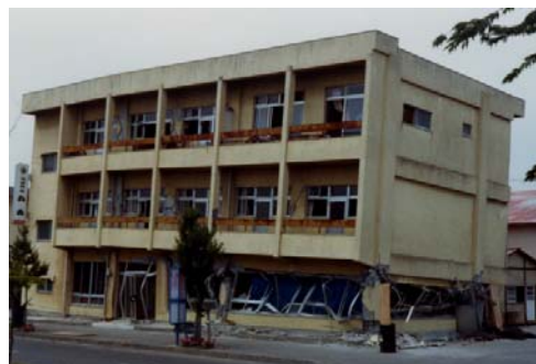
Collapse due to poor structural planning
