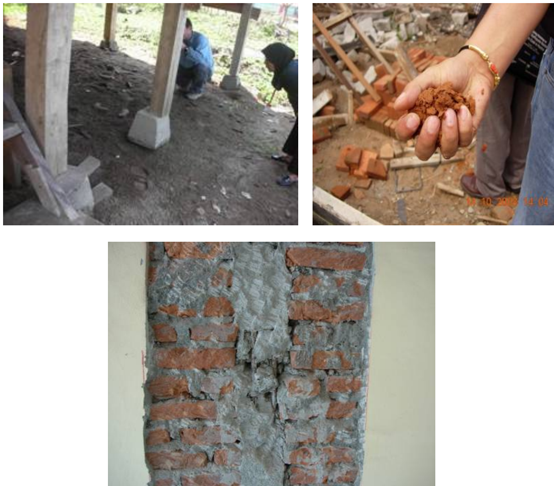
Figure 4. Problem in design, material quality and workmanship as observed in Aceh
