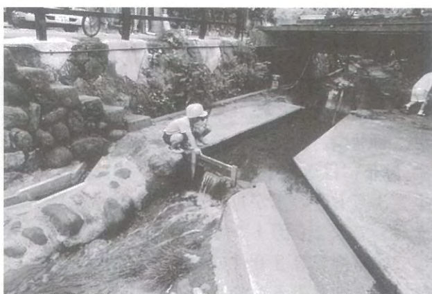
■ 1-61 Water flow is controlled by the wooden adjustment board at the diversion point.
