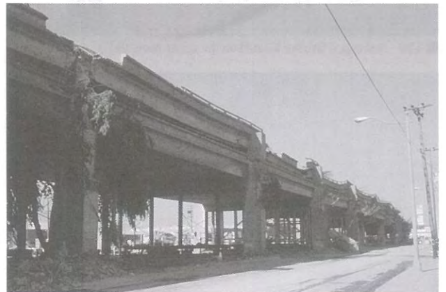
■ 1-35 Damage from the Loma Prieta Earthquake in 1989.
