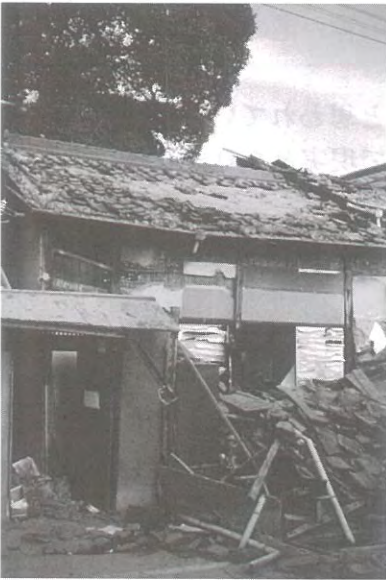
■ 1-4 Partly damaged wooden housing.
