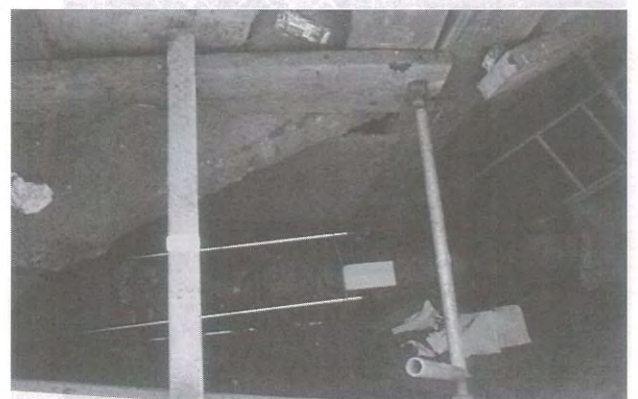
■ 1-28 Underground water-pipeline for exclusive use. (S.F.)
