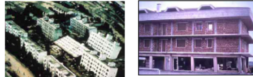
1. Failure of building due to liquefaction 2. Soft storey damage at ground floor
