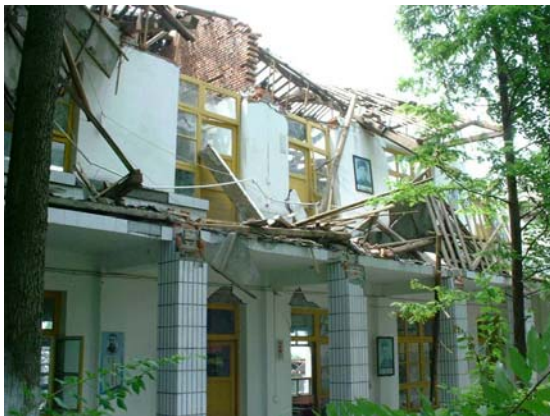
Figure 1.3 Damaged school building in Sichuan (June 2008)
