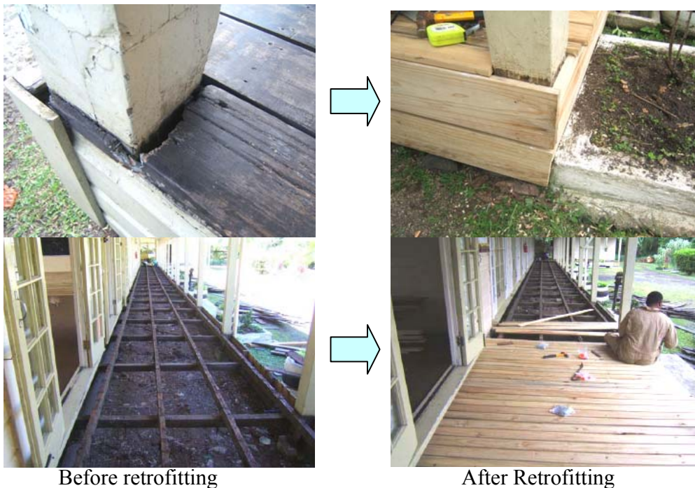
Figure 4.2 Example of retrofitting in Suva, Fiji
