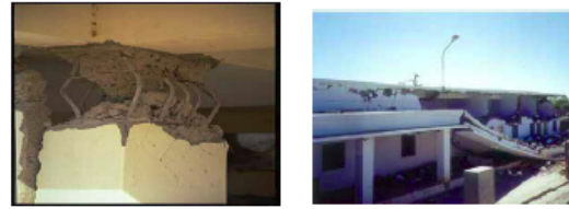
3. Failure of column-beam joint 4. Damage to school building in Gujarat (Poor configuration)
