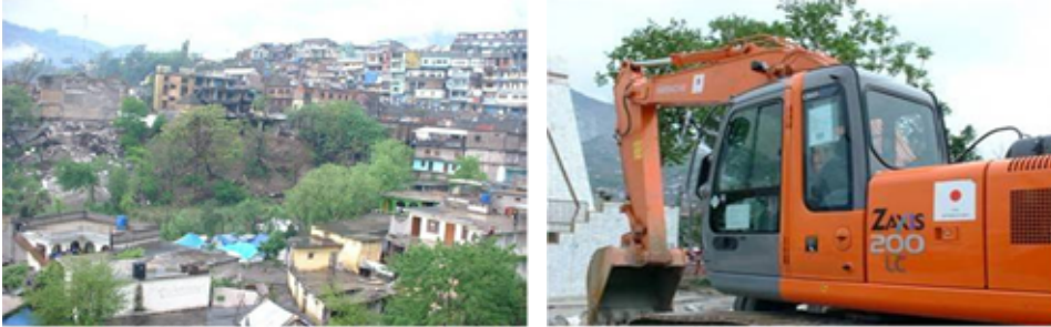
Figure: City of Muzaffarabad (Left) and the Operation of Reconstruction Works (Right), Muzaffarabad, Pakistan, March 2006
