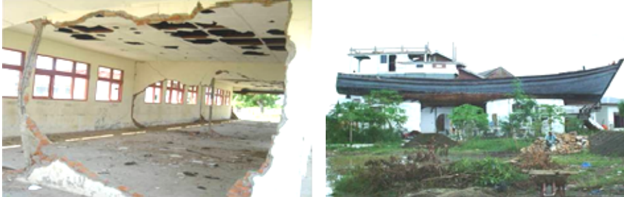
Figure: Damaged Masonry School (Left) and Remained Ship in the Residential Area (Right), Banda Aceh, Indonesia, December, 2007
