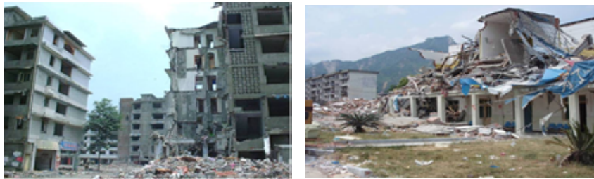
Figure: Damages in Middle Storey Apartment Houses- 5-6 Storeys Buildings (Left), Hospital in Hanwang (Right), Sichuan Province, China
