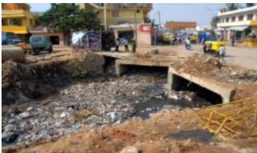
Chokes city drains
