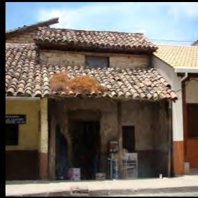
Buildings in bad condition
