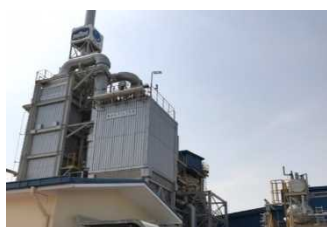
Waste to Energy Plant, JFE engineering, Myanmar
