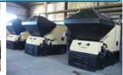
High-efficiency Heat only Boilers, Suuri-Keikaku, Mongolia
