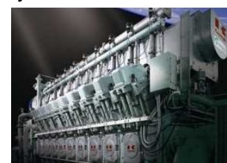
Co-generation system at factory, Toyota, Nippon Steel & Sumikin Engineering, Indonesia, Thai
