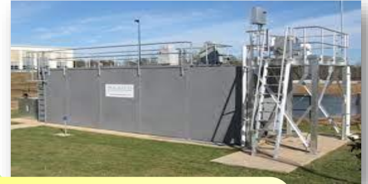
Japan Sewage Works Agency Teijin's Multi-Stage Activated Biological Process technology (MSABP)
